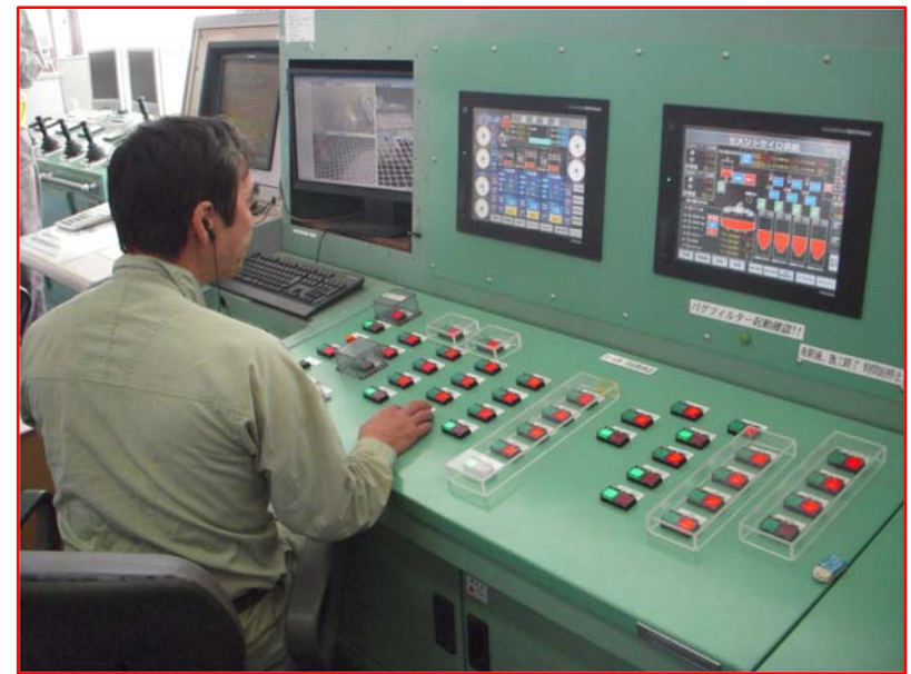
Control room inside the ship
